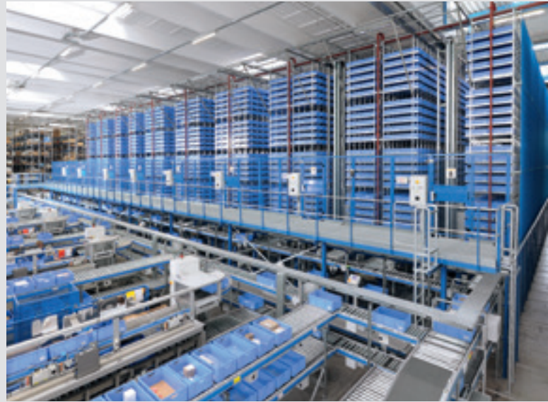
▲ LTBs catapult automated warehouses into the premier league
